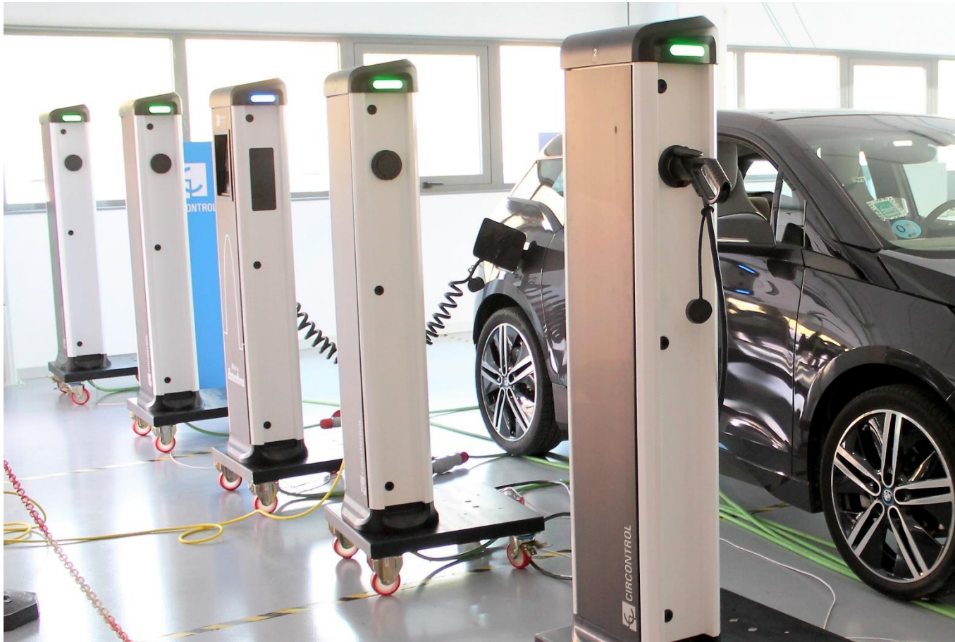
(master-slave system at Circontrol laboratory)
